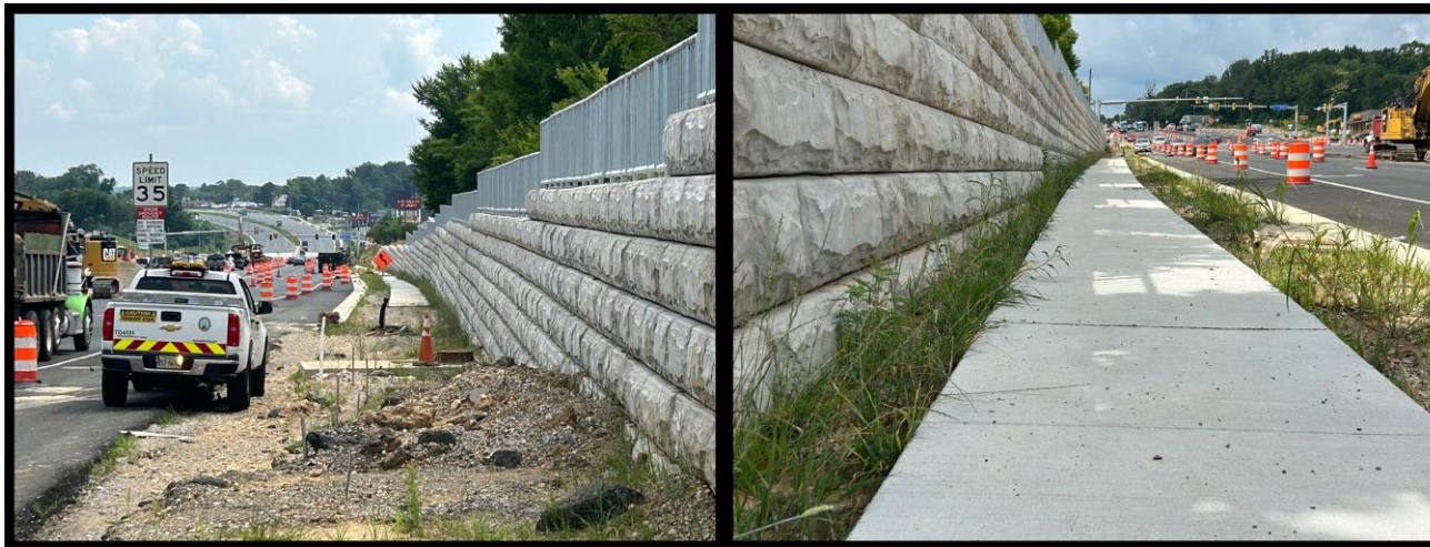
Sidewalk install completed and installation of the Ornamental Streetlighting has been authorized.
