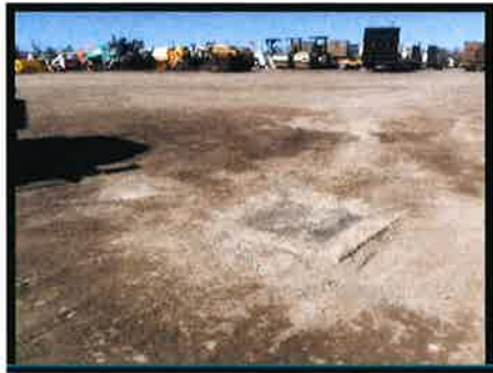
Unprotected drop inlet
