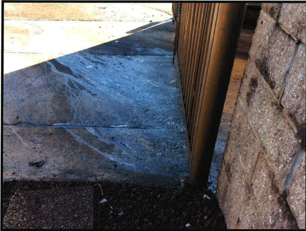
Figure 1: Photo of Discharge.
