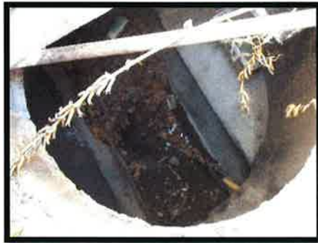
Debris at Manhole D
