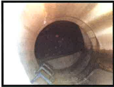
Debris at Manhole A
