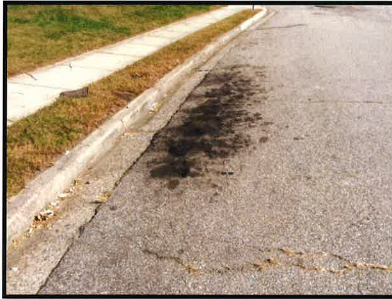
Figure 1: Photo of Discharge.
