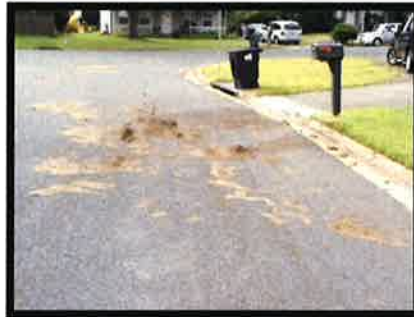
Figure 1: Photo of Discharge.
