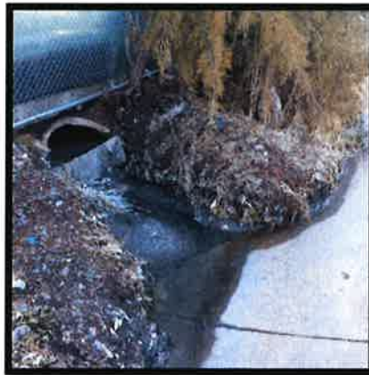
Figure 1: Photo of Discharge.
