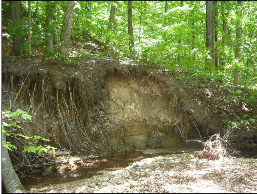
Photo 112: Localized streambank erosion on the outside of a meander on Reach 630-C.
