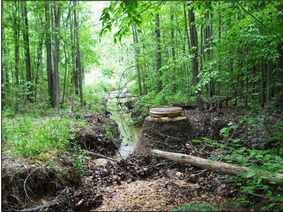
Photo 27: Channel erosion and exposed sanitary sewer along Reach 630-D.
