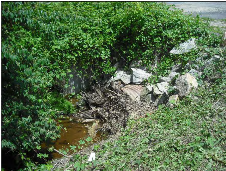
Photo 484: Debris clogging the CMP culvert at the downstream end of Reach 645-A.
