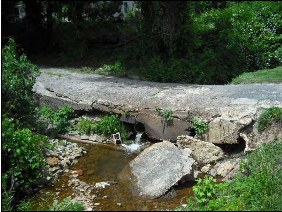
Photo 471: Paved low water crossing in poor condition, along Reach 645-A.
