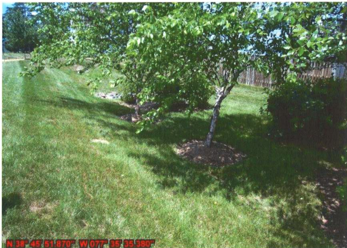
Photo 2 (364): Typical example of “Bioretention” facility lacking detention
