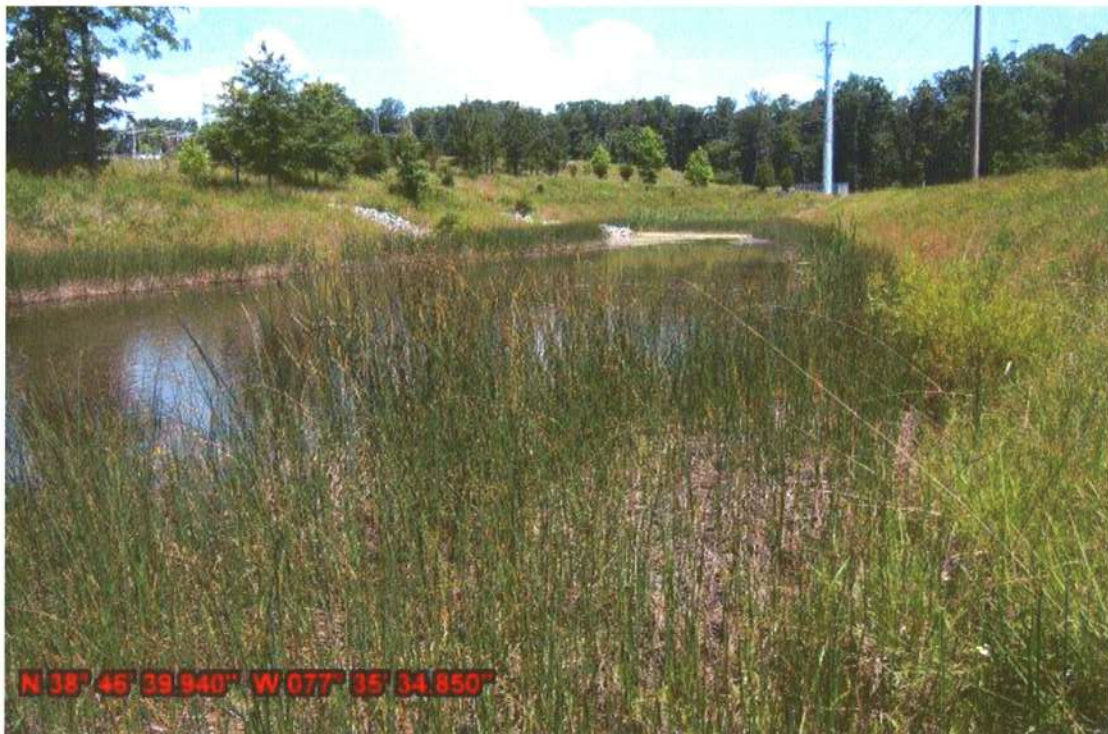
Photo 2: Sediment accumulation visible in background
