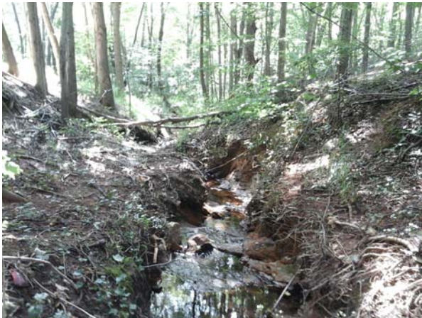
Highly eroded outfall channel surrounded by dense tree cover.
