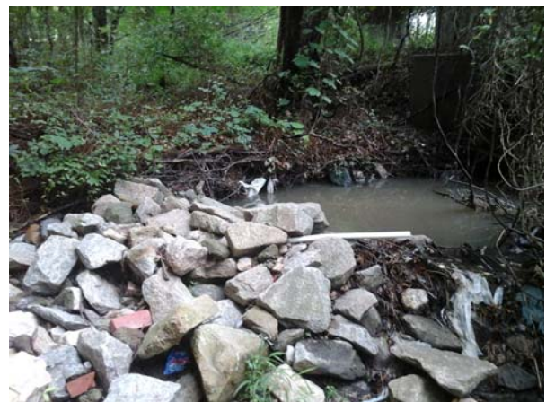
Pile of rip rap just downstream from the plunge pool and opening of outfall pipe.
