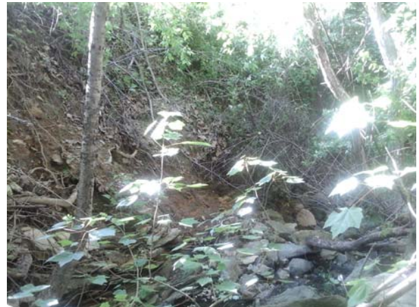
Severely erosion in the outfall channel and steeply sloped banks surrounding the channel.
