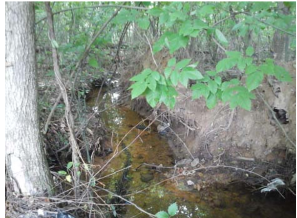
Severely eroded channel just downstream from the outfall pipe, with near vertical banks and trees surrounding the channel.
