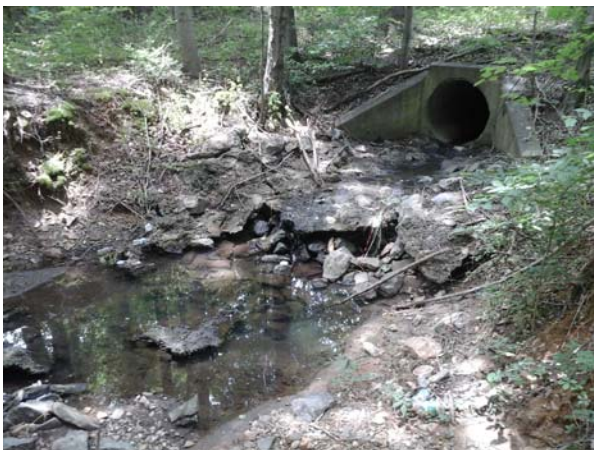
Outfall pipe with crumbling concrete deck, falling into the highly eroded channel.
