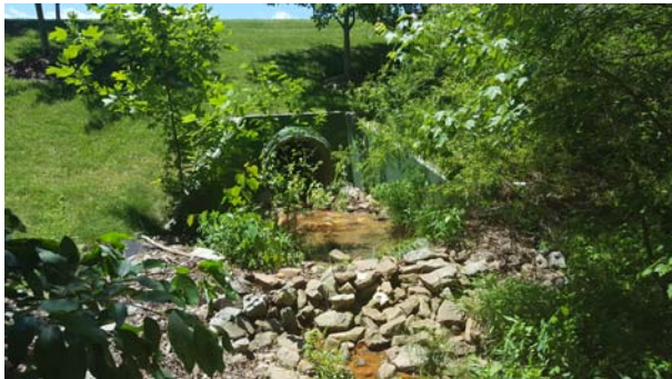
Outfall pipe and remaining rip rap/armor at the head of channel.
