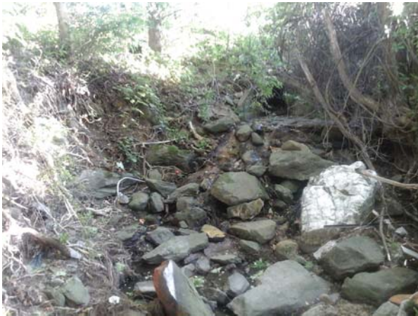
Severely eroded outfall channel and dispersed boulders just downstream of the pipe.
