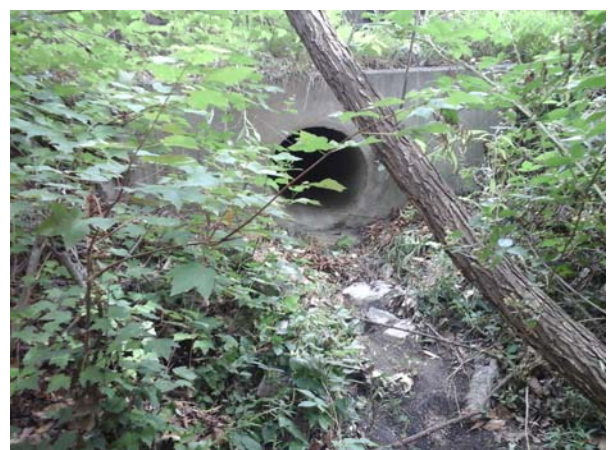
Upstream view of the outfall pipe, surrounding vegetation and beginning of the steep channel are visible.
