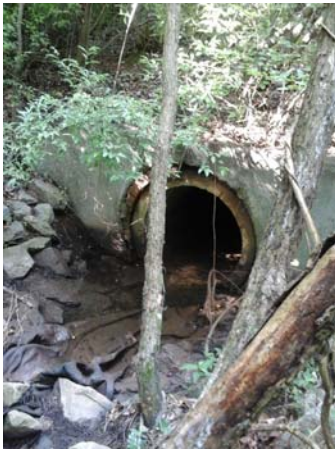
Stream channel downstream of outfall, flocculent heavily present and erosion visible.
