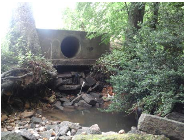
Upstream view of the outfall pipe, pipe deck completely gone and erosion visible in the receiving channel.
