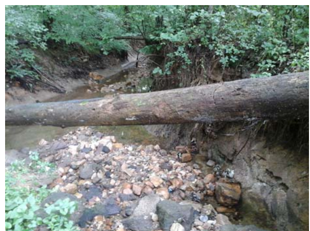
Downstream view of the outfall channel, wooded banks and severe erosion visible.
