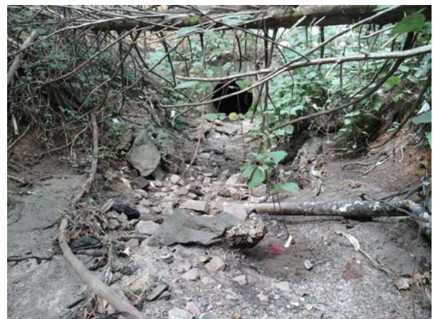
Downstream view of the outfall channel leading to the stream channel; erosion is less severe further downstream.
