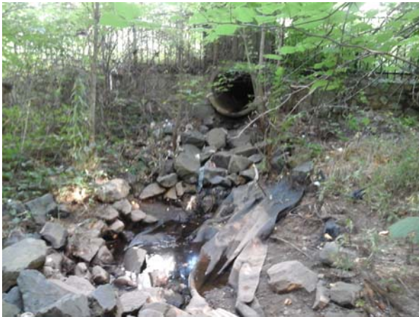
Upstream view of the outfall pipe, steep slope and drop into the channel visible.
