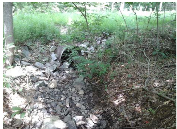
Upstream view of the outfall pipe and remnants of rip rap and concrete deck.
