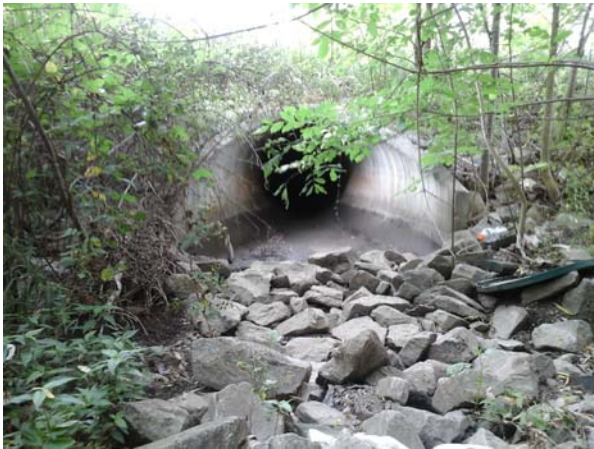
Upstream view of the outfall pipe itself, heavy vegetation and rip rap present.
