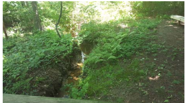
Heavily eroded channel just downstream from the outfall pipe and failing armor.
