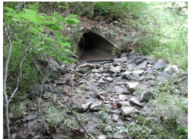
Upstream view of the outfall pipe and remaining rip rap at the opening.
