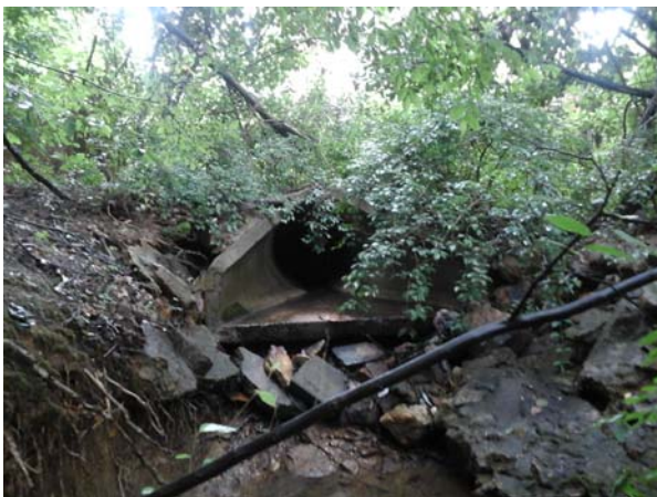
Upstream view of the outfall pipe and remaining pieces of the pipe deck. High levels of degradation are visible from the discharge
