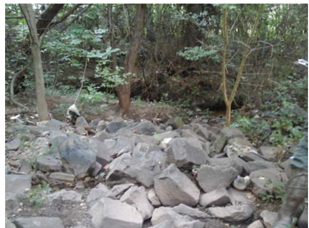
Downstream view of confluence of outfall and stream channel. Moderate erosion and steep slope visible.
