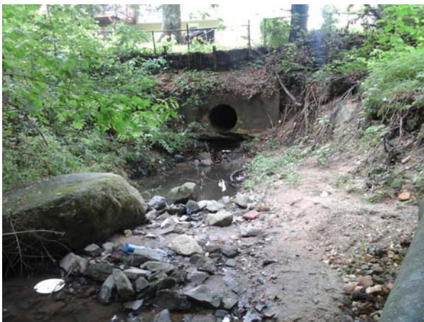
Upstream view of the outfall pipe, drop into channel is visible as well as the steep drop off on the property.
