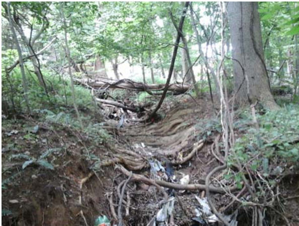
Upstream view of the outfall pipe and the eroded area immediately downstream of the pipe.
