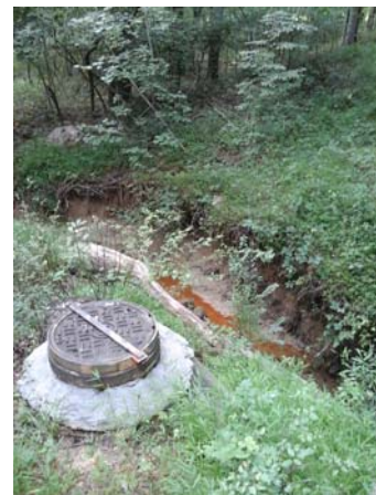
Sanitary manhole directly adjacent to highly eroded outfall channel.
