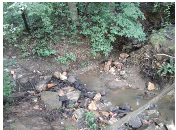
Outfall channel just downstream of the pipe opening, highly eroded banks and tree cover is visible.
