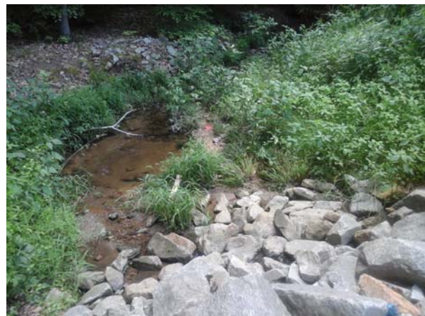
Receiving channel receiving uncontrolled stormwater from outfall
