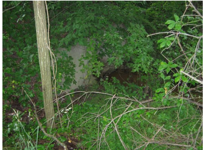
SWM BMP outlet inside SWM facility
