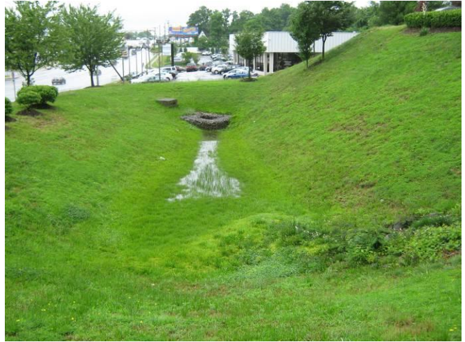
Overview of primary riser and low flow orifice structure from the driveway.
