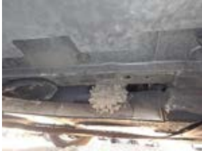
View of Plug N Dike on cracked fuel tank.
