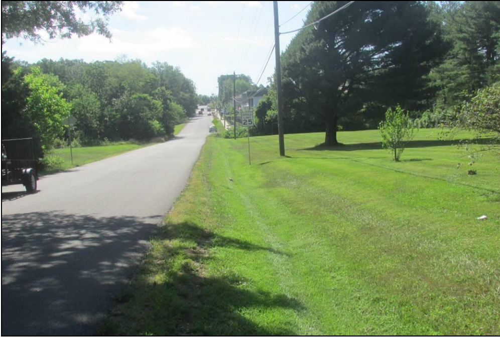
Photo 7: Drainage Ditch Occupying Entirety of Project Area Along Jennell Drive, Looking East.
