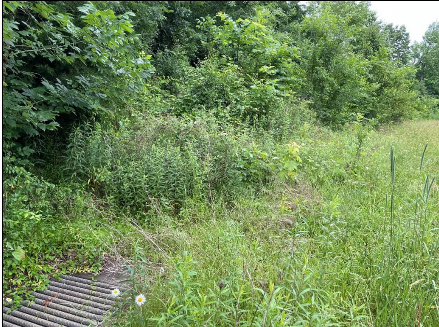
Photo 5: Storm Sewer and Steep Grade Along West Side of Devlin Road, Looking North.
