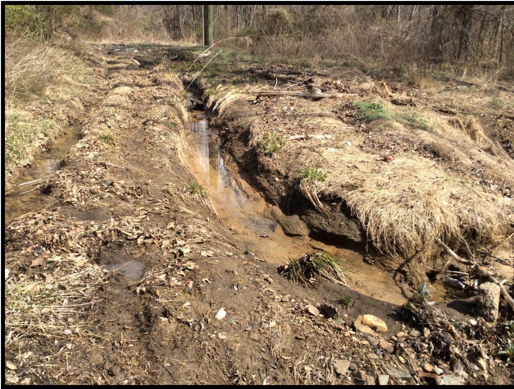
Erosion made by flood at vehicular track and diverted towards river
