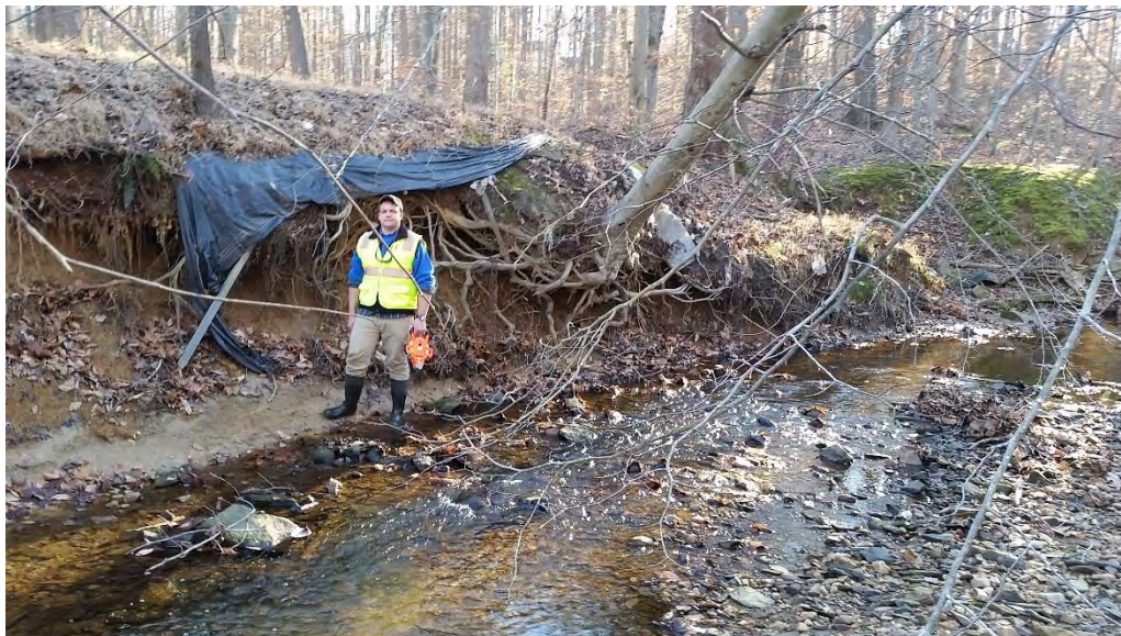
Figure 9: Stream bank incision >6 feet (vertical instability) from bed. Photo was taken downstream from sampling reach.
