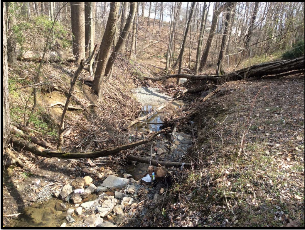
Erosion at downstream channel
