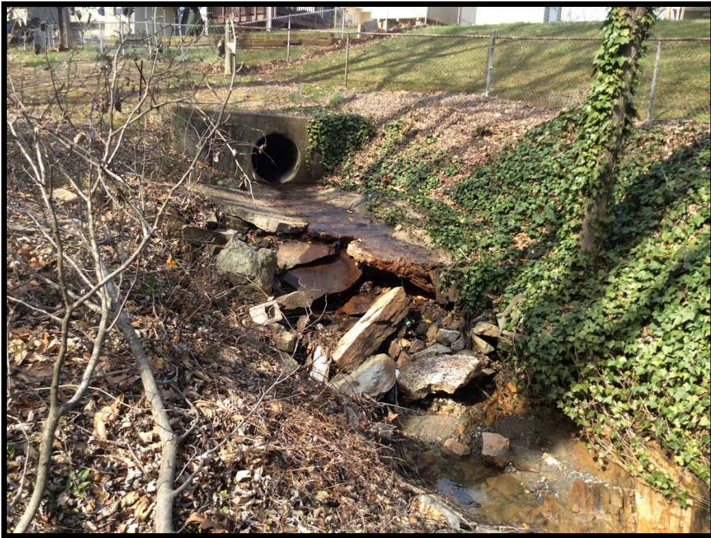
Erosion at downstream channel
