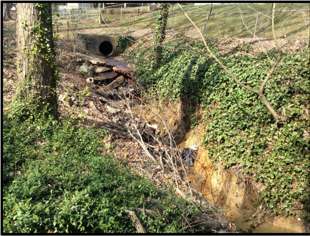
Erosion at downstream channel
