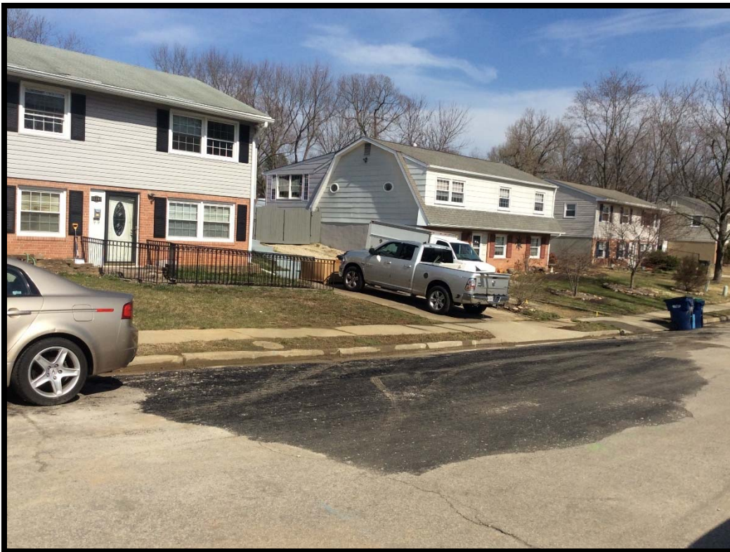
Location of Maintenance of Unusual Discharge (15107 Calexico Ln)
