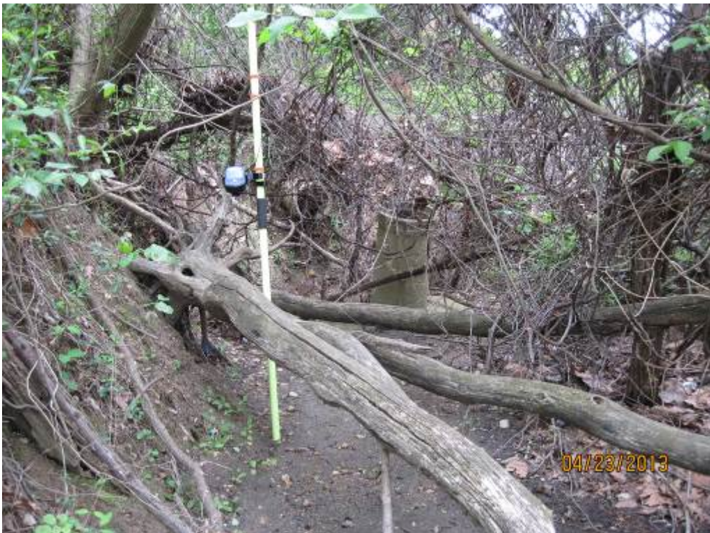
56. Looking upslope at a failing section of pipe adjacent to Stream Reach 18A. The pipe has undercut itself and the end-section has fallen off.
