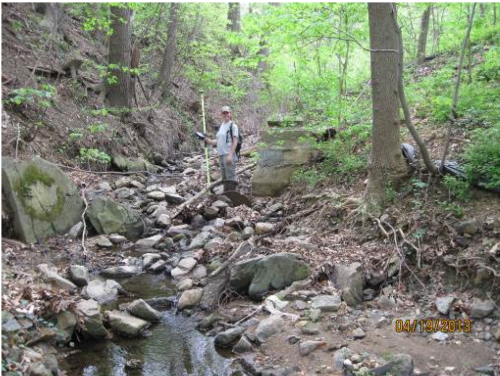
52. Looking upstream at a typical section of Stream Reach 17A. This section is somewhat incised, partially exposing at least one sanitary sewer line.
