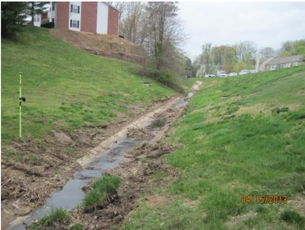
70. Looking upstream at a concrete channel that concentrates water into Stream Reach 20B.
