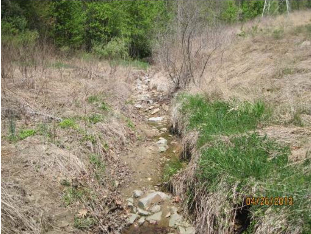
35. Looking upstream at a portion of Stream Reach 10 within a powerline easement. This section is significantly aggraded due to upstream erosion.
