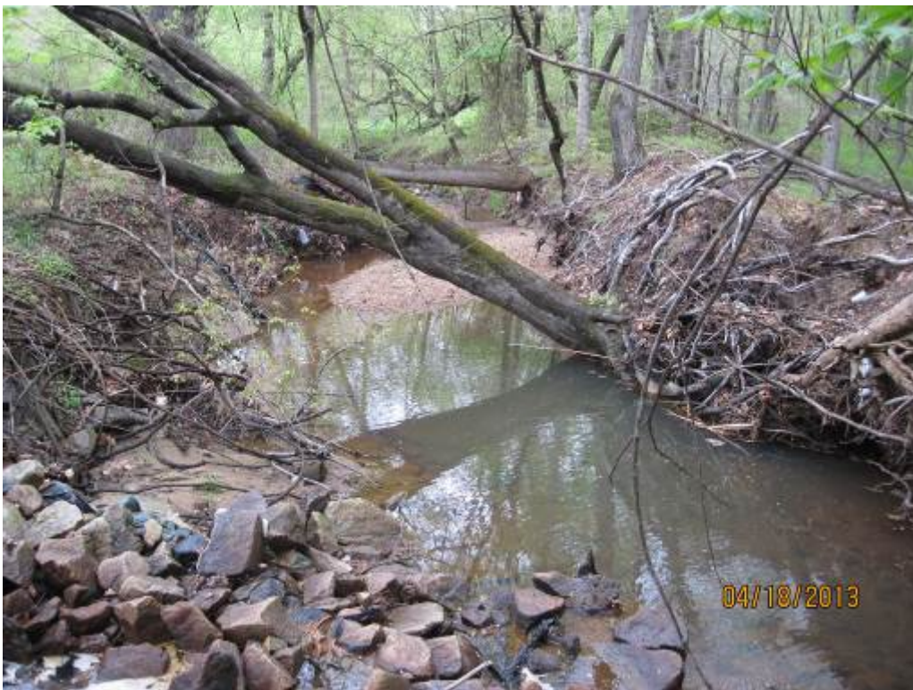
78. Looking downstream at a typical section of Stream Reach 23. This stream is unstable, with significant erosion and undercutting.
