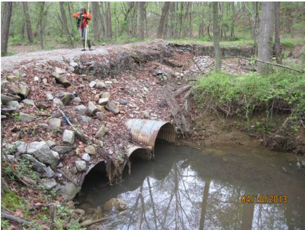
80. Looking upstream at the downstream end of Stream Reach 23, where a sanitary sewer line crosses above the stream and the corrugated metal pipes. This area has been stabilized with gabion baskets, which have shifted the areas of erosion. This area could be compromised in the future.
