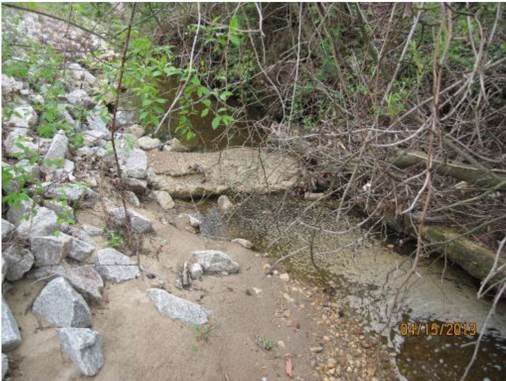
64. Looking downstream at an exposed utility within Stream Reach 19B. This stream has been significantly altered in order to stabilize the left bank, along Devils Reach Road.
