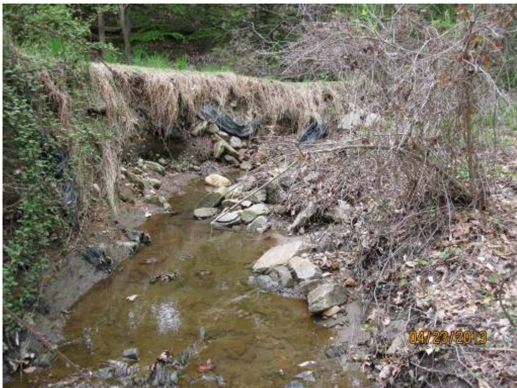
58. Looking upstream at a typical section of Stream Reach 18B. This stream is incised with areas of instability throughout.
