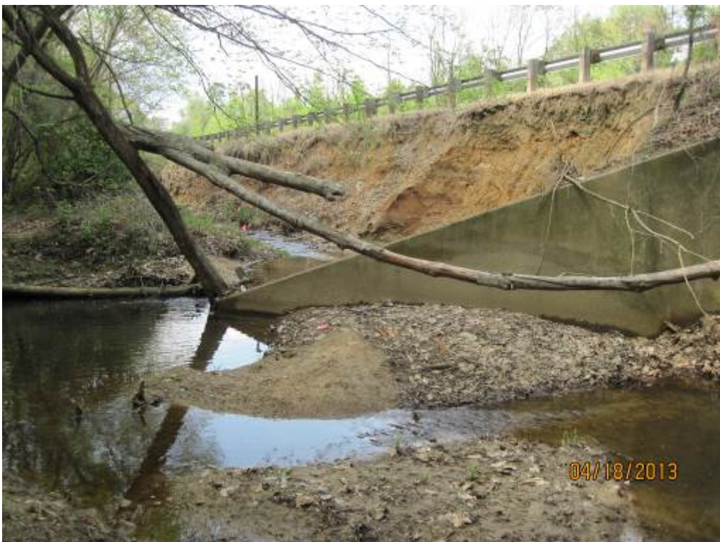
74. Looking upstream at the downstream end of Stream Reach 21. This section is severely eroding behind the wing-wall under a ramp for I-95. This stream poses a danger to the ramp itself.
