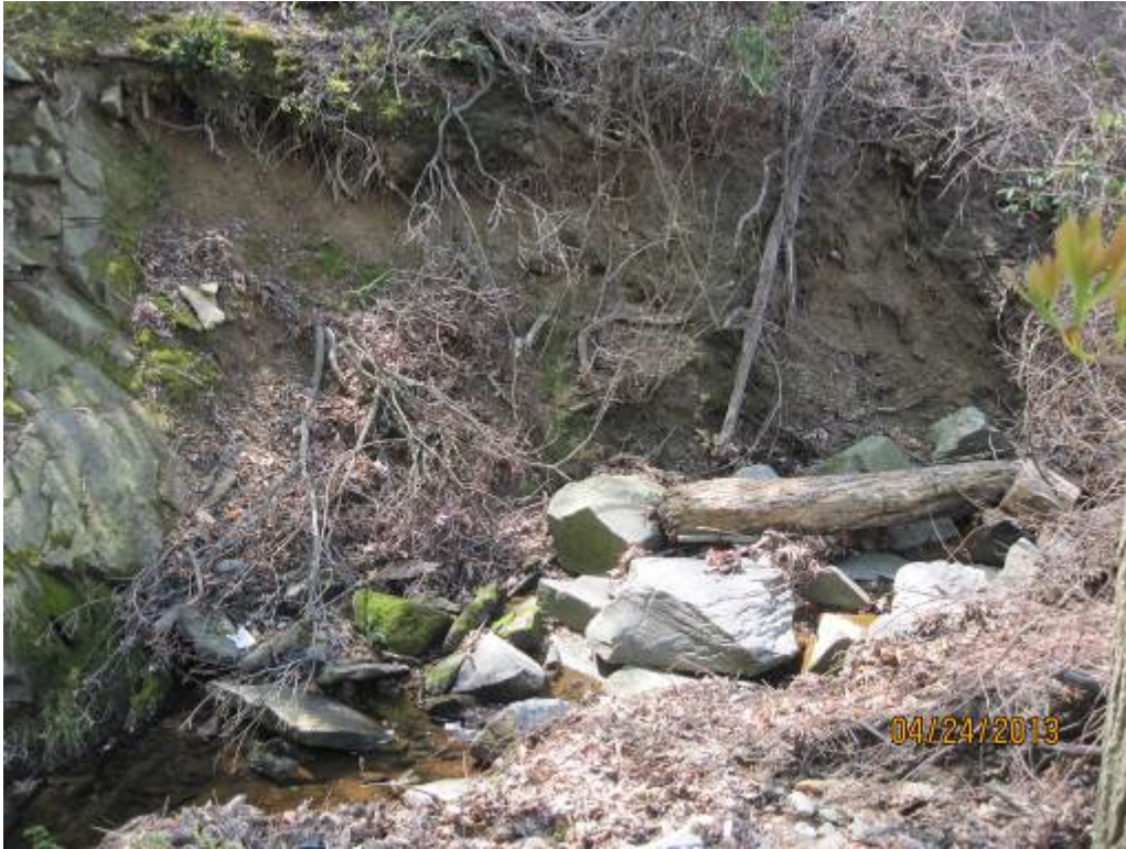
13. Looking upstream at a severely eroding bank downslope of a stormwater pond outfall located on-line with Stream Reach 5.
