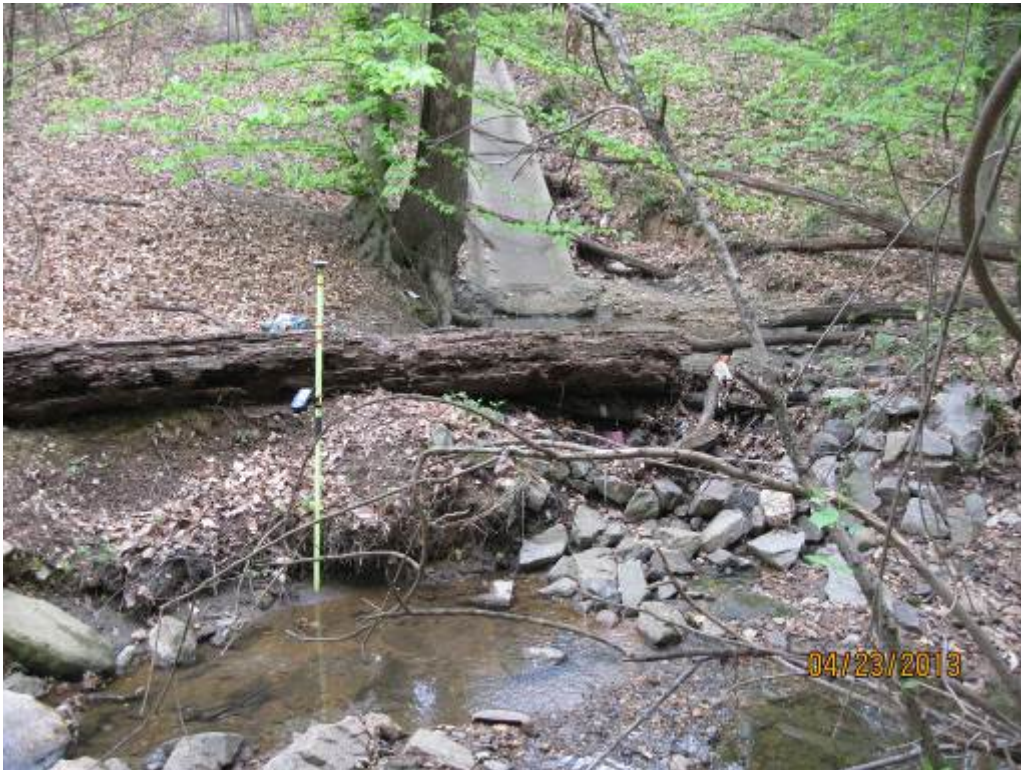
59. Looking upstream at a concrete flume that carries stormwater to Stream Reach 18B. These flumes are likely responsible for at least some of the erosion seen in this channel.
