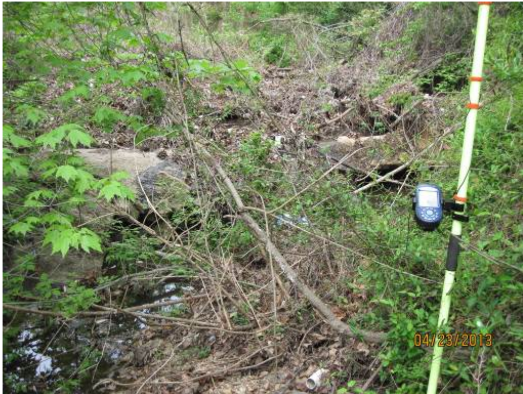
57. Looking upstream at an exposed sanitary sewer line in Stream Reach 18A. This utility is beginning to be undercut, with the possibility of future failure.
