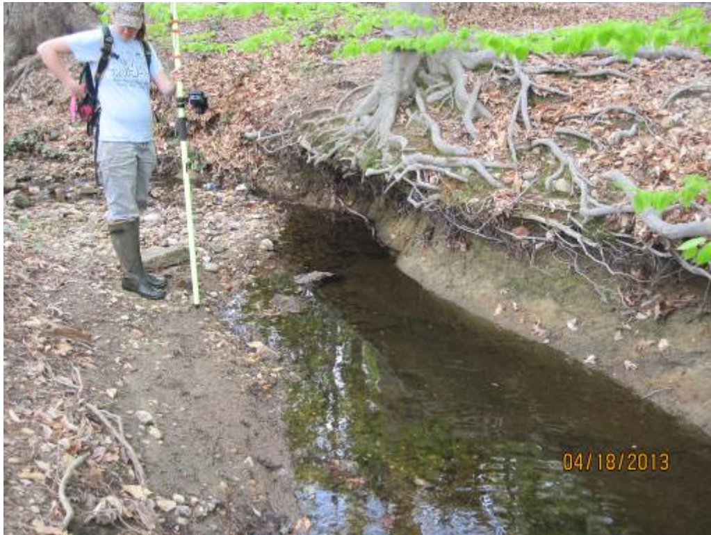
75. Looking downstream at a typical section of Stream Reach 22. This stream reach typically shows incision on one side of the channel.
