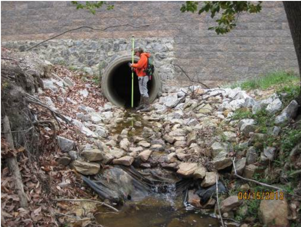
61. Looking upstream at Stream Reach 19A. The end of the rip-rap channel lacks a stable transition to the stream channel, and is starting to fail.
