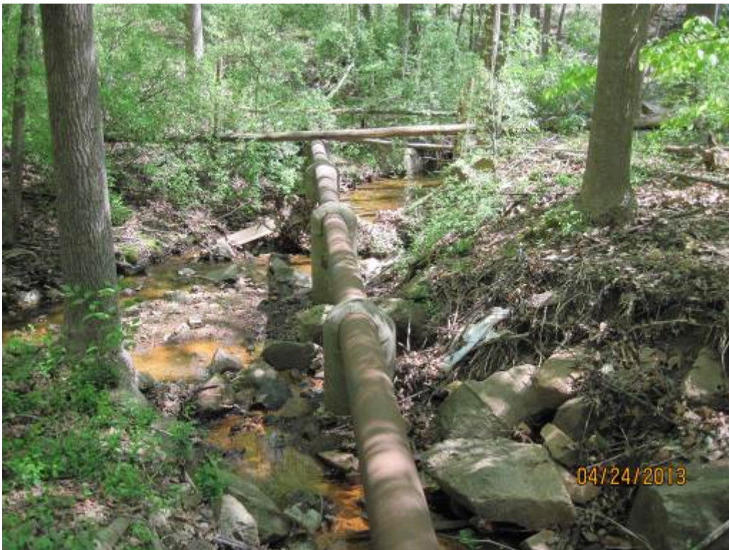
12. Looking downstream at an elevated utility crossing over Stream Reach 5. Some erosion is present around these piers.
