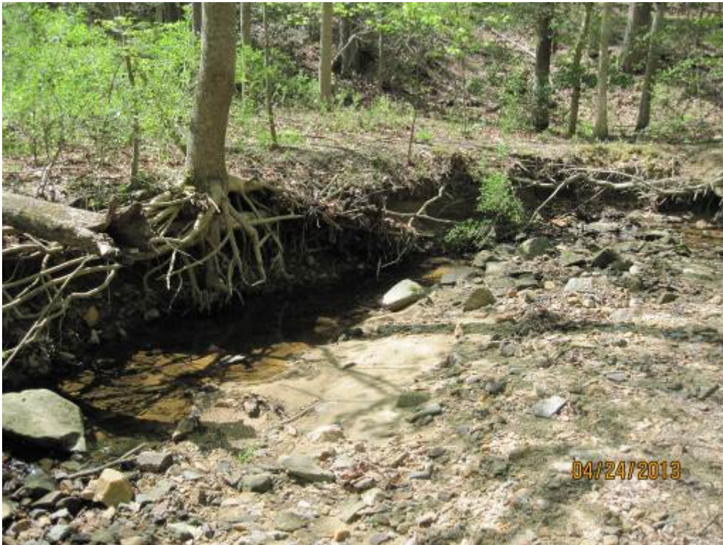
11. Looking upstream at a streambend showing some significant erosion in Stream Reach 4.
