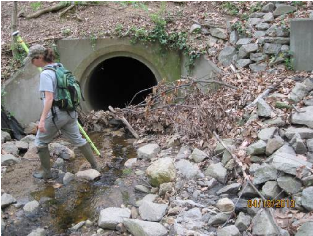
53. Looking downstream at Stream Reach 17B. The downstream portion of the channel is aggrading near this culvert.
