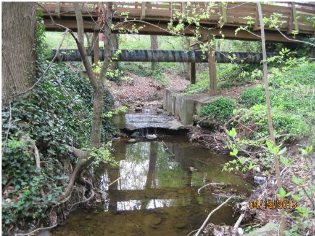
76. Looking upstream at a utility crossing over Stream Reach 22. The concrete apron is starting to undercut.
