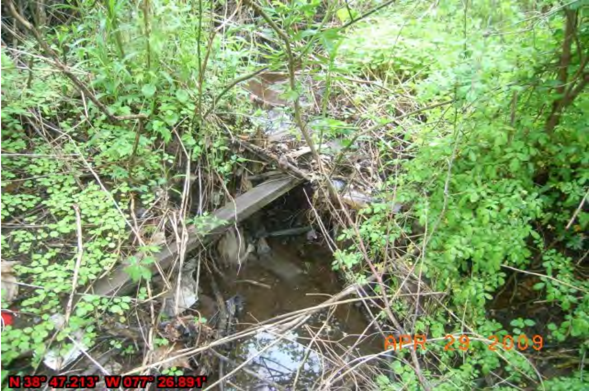
Photo 2: Stabilize headcut Y7-H1
