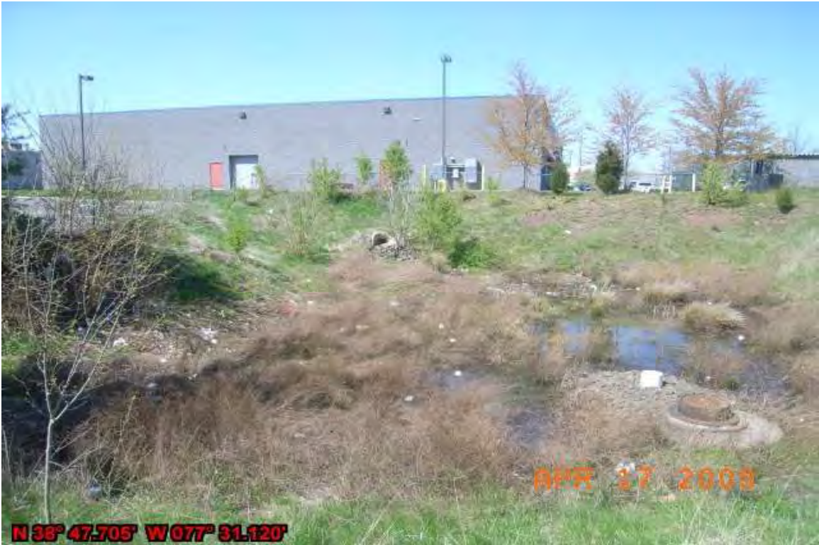
Photo 1: Showing lack of maintenance and inadequate riser
