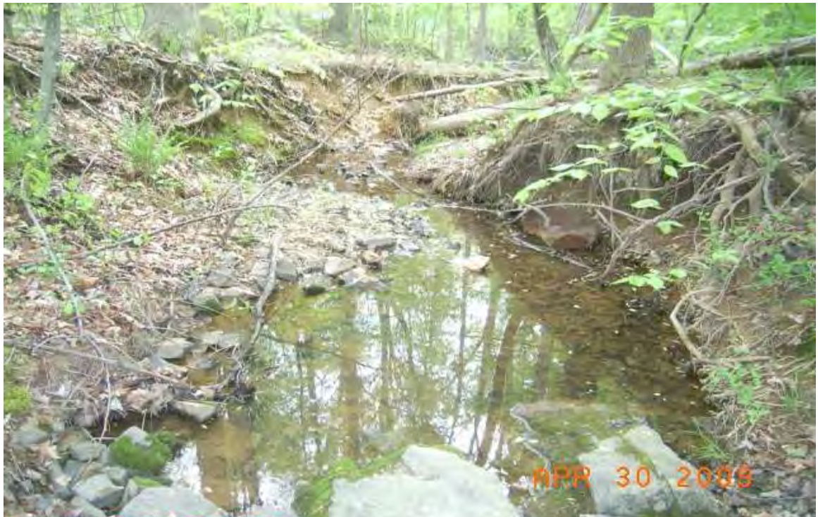
Photo 1: Scour and erosion is evident downstream of BMP outlet
