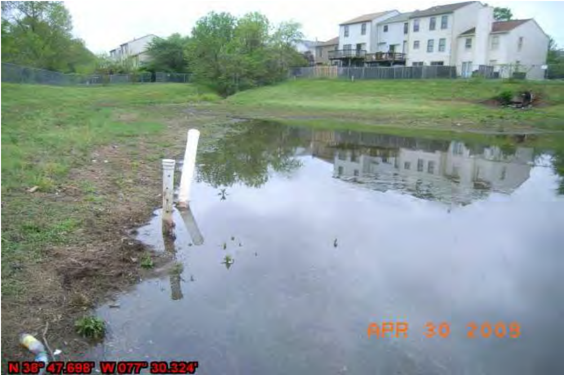
Photo 1: Low flow orifice for dry basin is clogged and not connected to riser
