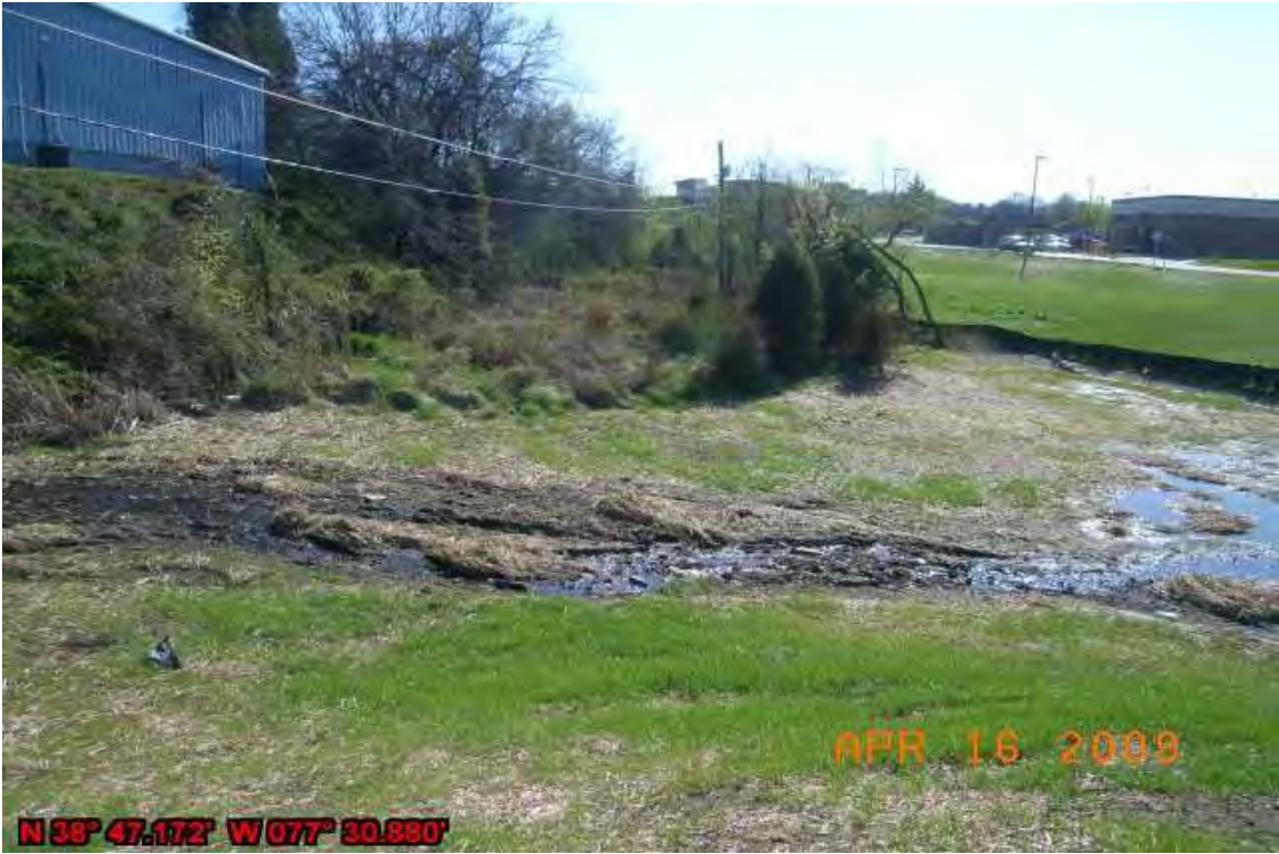
Photo 1: Outfall without adequate channel creating erosion
