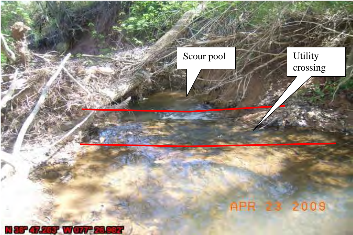
Photo 1: Utility crossing scour on downstream side
