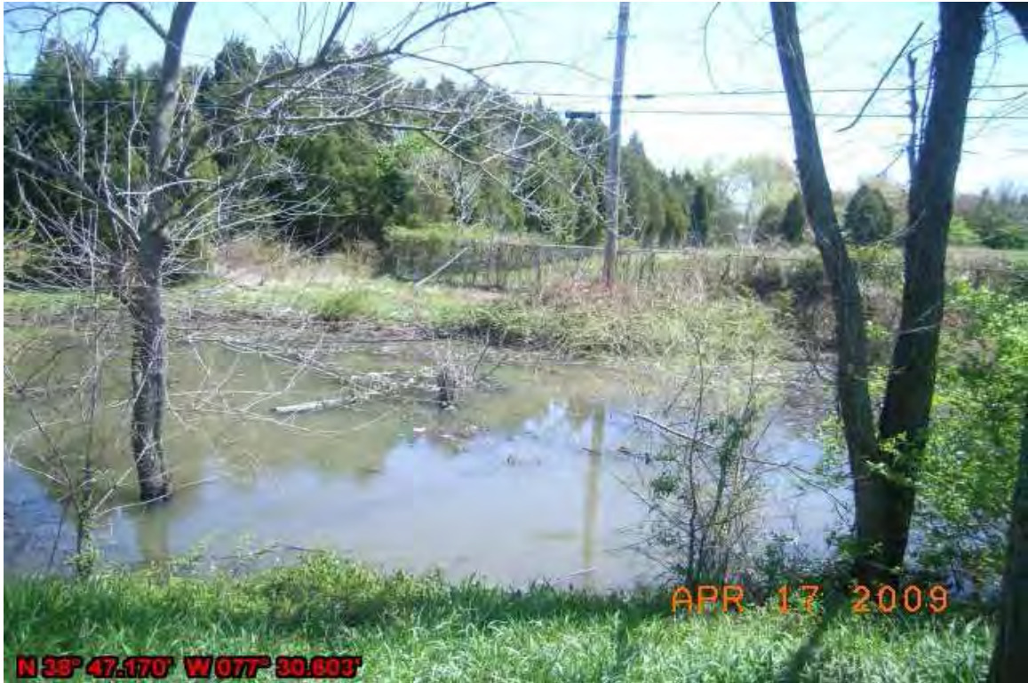
Photo 1: BMP 166-2 is a poorly functioning stormwater facility
