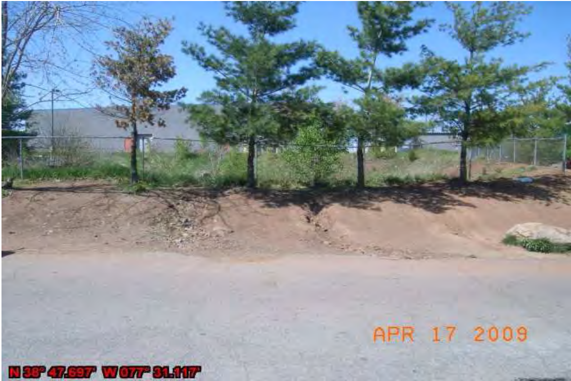
Photo 2: Erosion along backside of berm
