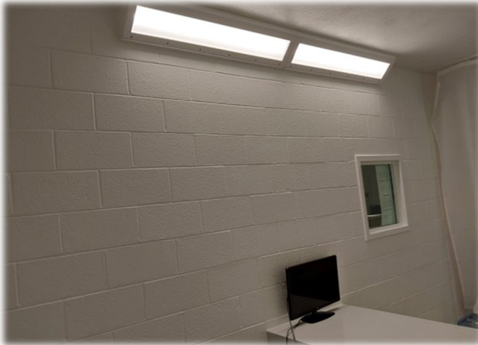
New lighting fixtures in the day room
