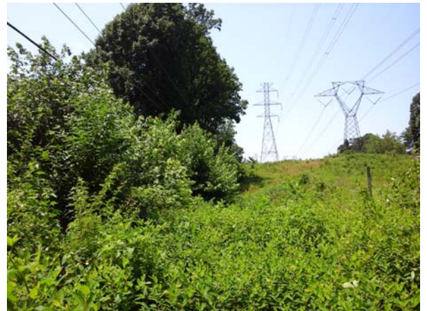
View looking southeast through the electric transmission line ROW at site UFOR137.
