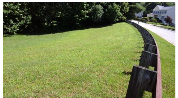
View looking north (parallel with slope) along a buried culvert area at site RFOR109.
