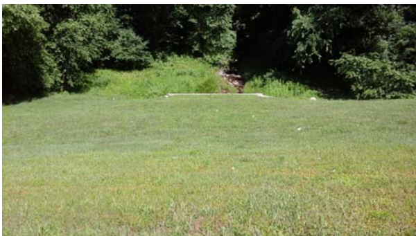
View looking northwest (downslope) along a buried culvert area at site RFOR109.
