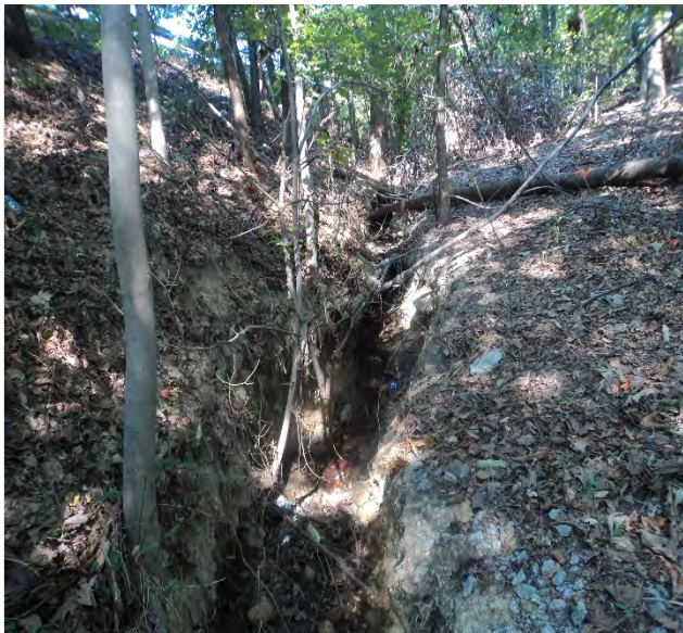
Photo 23: deeply incised upland roadside toeslope ditch, N. side of Opitz Blvd at E end of project.
