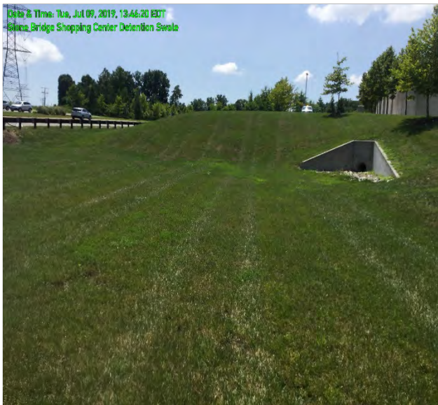
Photo 3: Stormwater dry detention basin at Bridge View Way intersection w Potomac Center Boulevard. Upland area.
