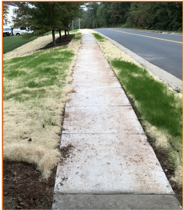
Godwin Drive Sidewalk – This project completed a missing section of sidewalk on Godwin Drive adjacent to Lancaster Knoll Lane.
