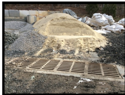
unprotected drop inlet
