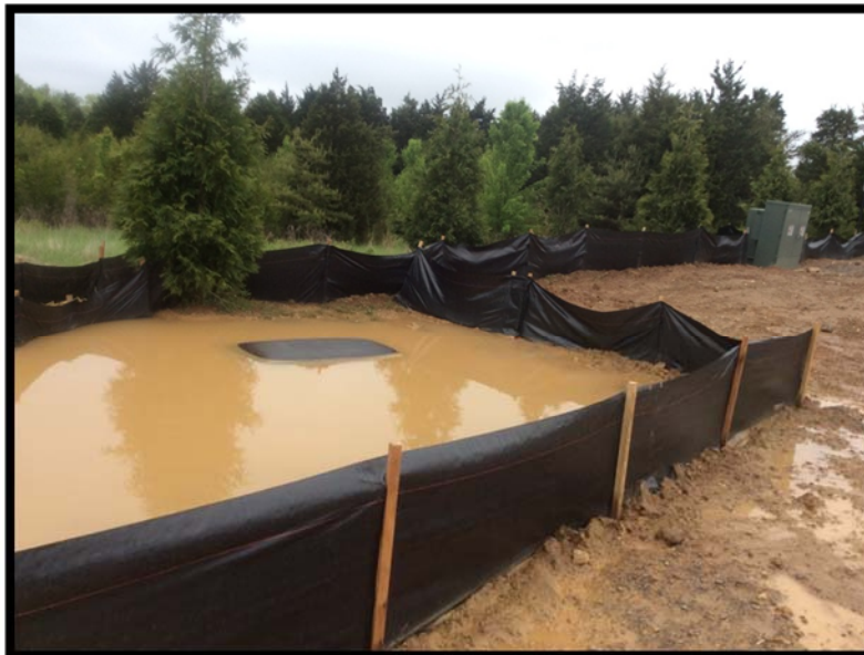
Zone -2 (Silt fence around outlet of settling basin with mud bag)
